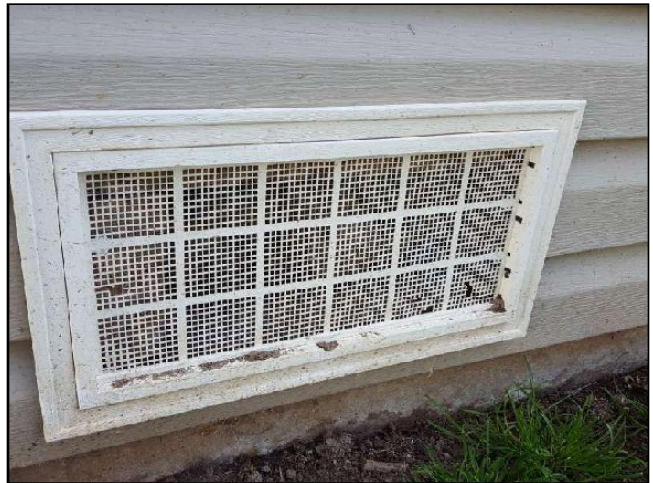
Vent screens damaged
