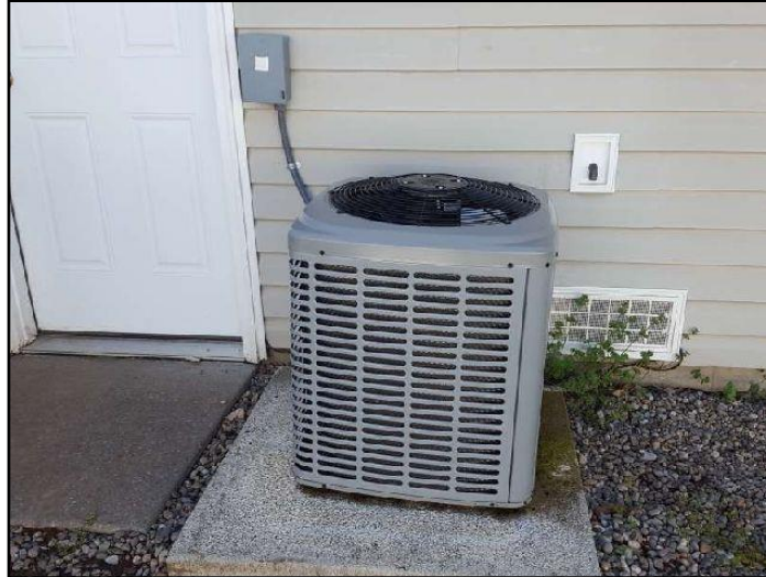
Central air conditioner
