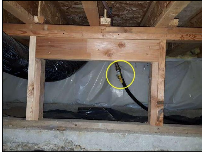
Main water shut-off valve
