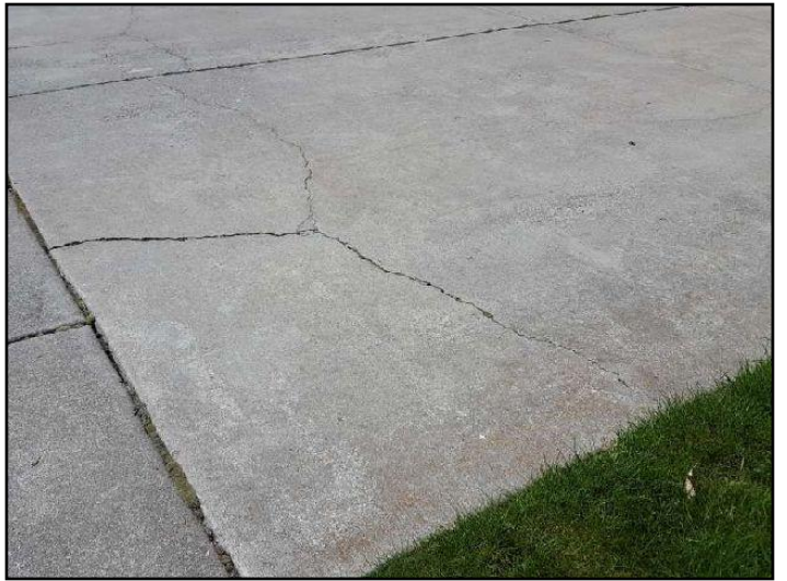
Cracked or damaged surfaces
