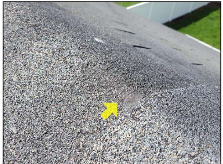
Granule loss on ridge
