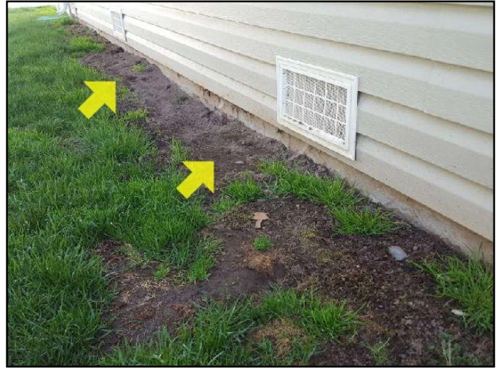
Improper slope or drainage
