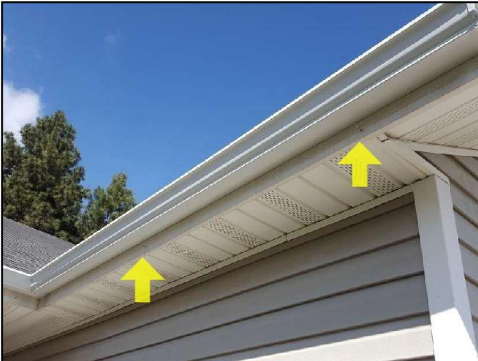
Hooks and holes in fascia
