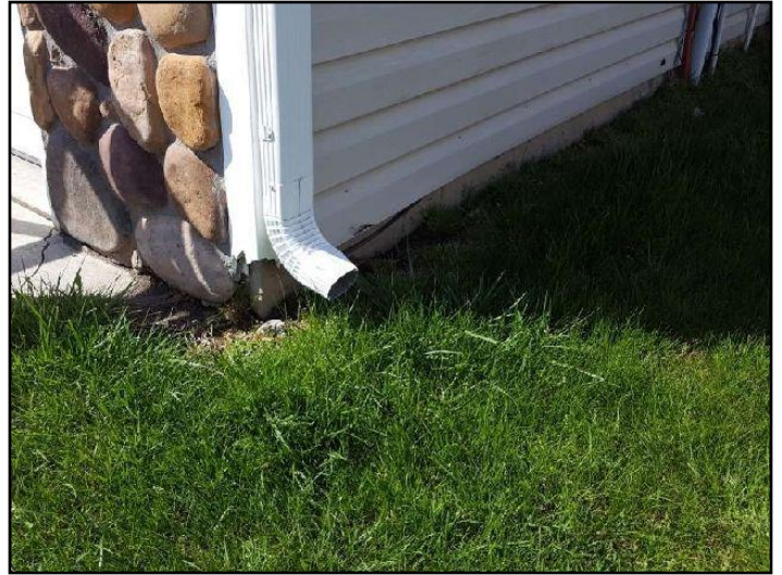
Discharge too close to building
