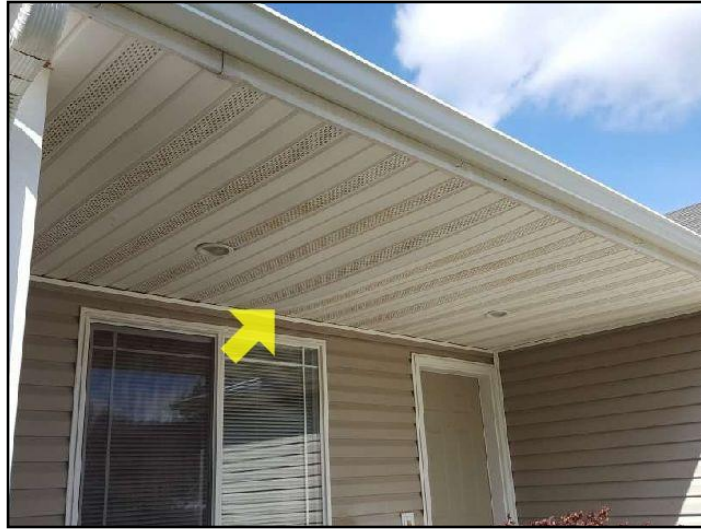
Loose soffit trim
