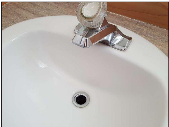
Drain stop missing
