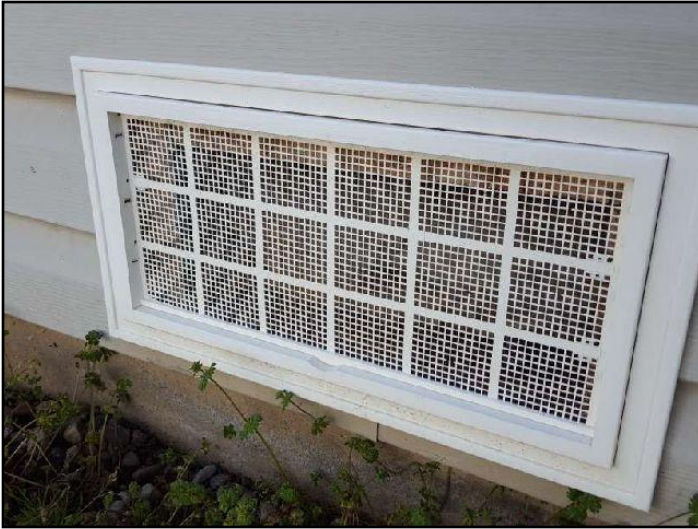
Missing vent covers
