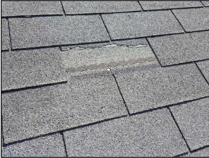
Missing shingle tab
