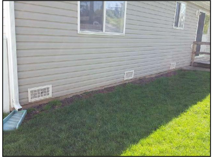
Missing vent covers
