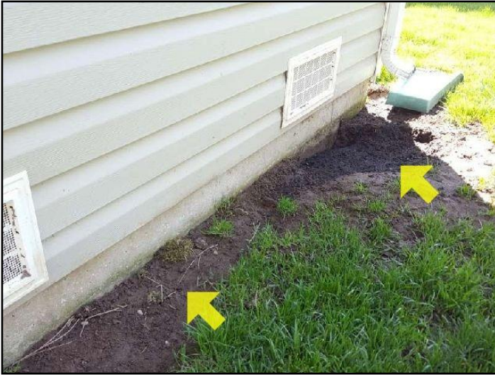
Improper slope or drainage
