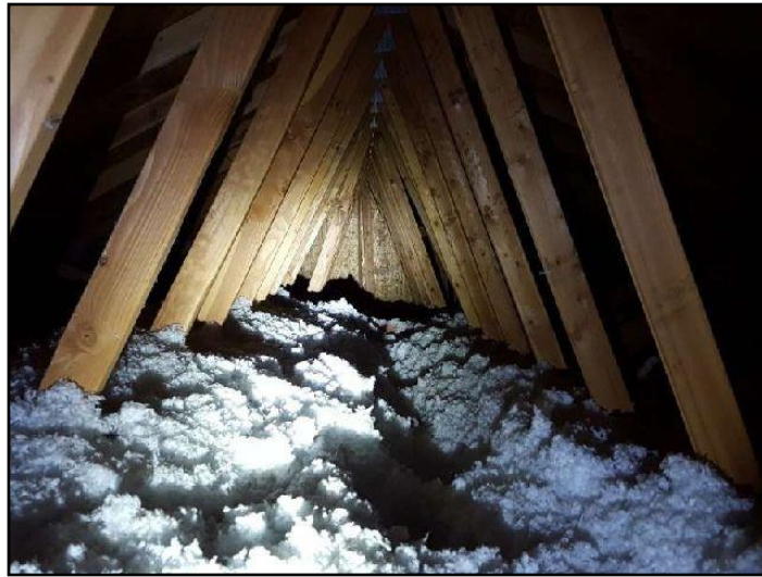
Foot traffic has compressed insulation
