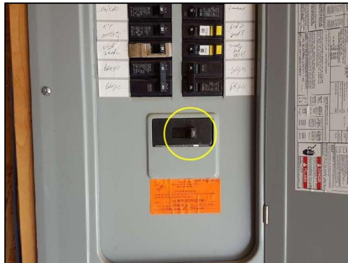
Main electric disconnect
