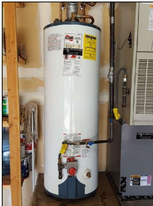
Gas water heater
