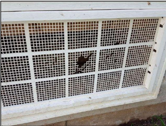
Vent screens damaged
