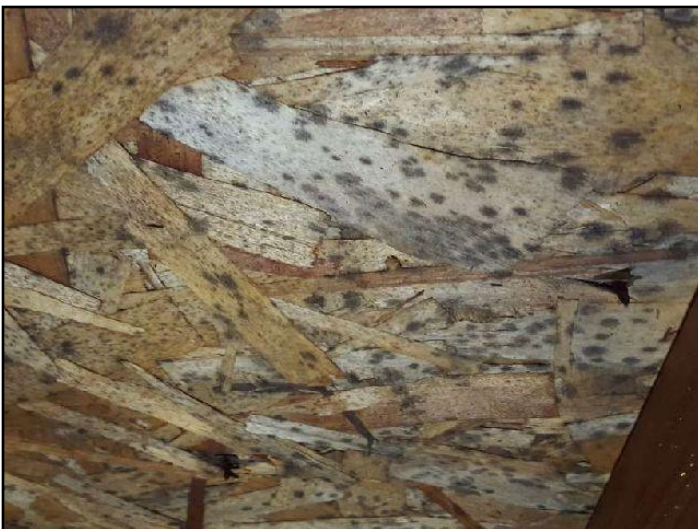
Possible mold/mildew Possible mold/mildew
