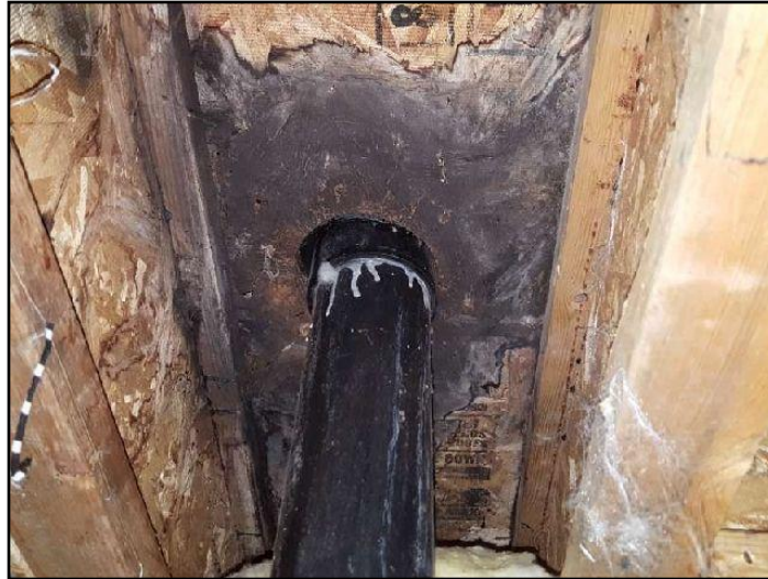
Wood rot / moisture damage
