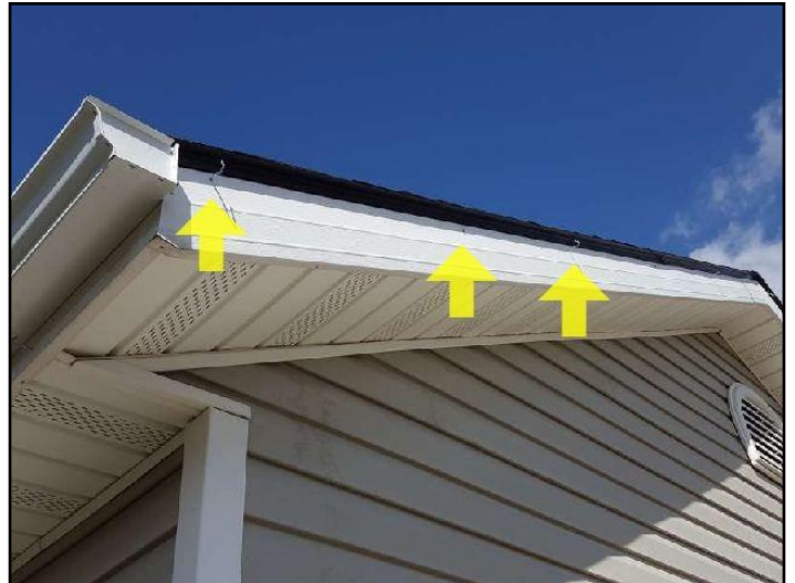
Hooks and holes in fascia
