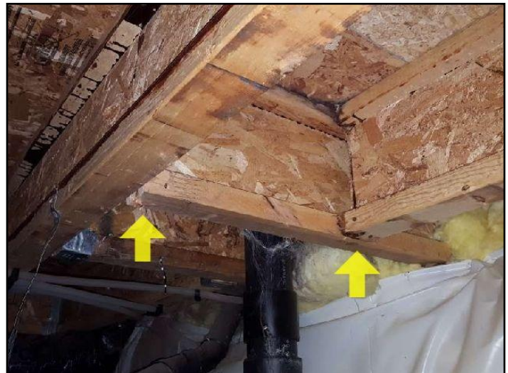
Missing joist hangers
