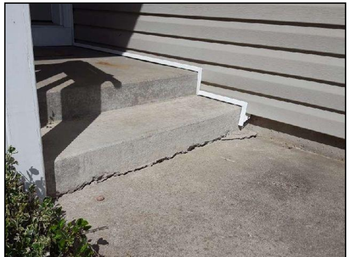
Cracked or damaged surfaces
