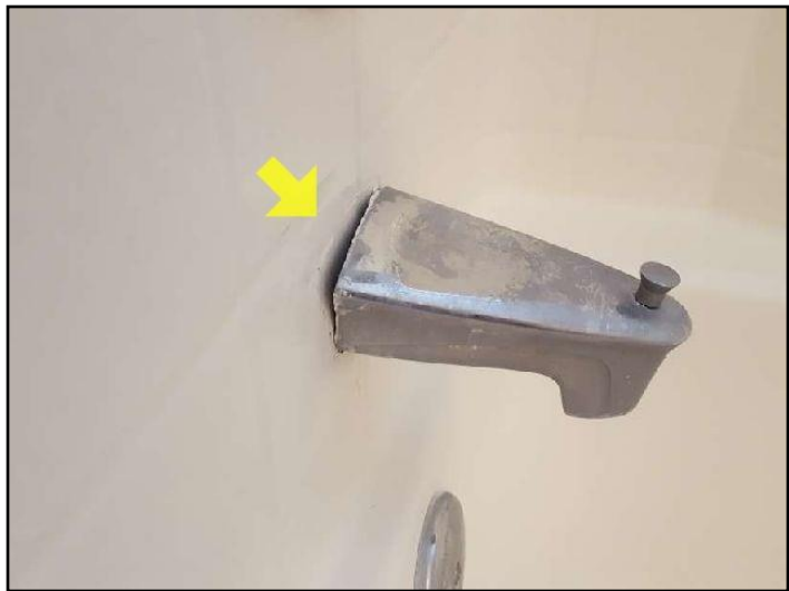
Faucet bent and separated
