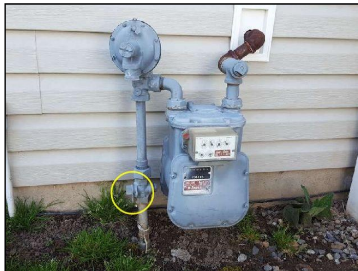
Main gas shut-off valve
