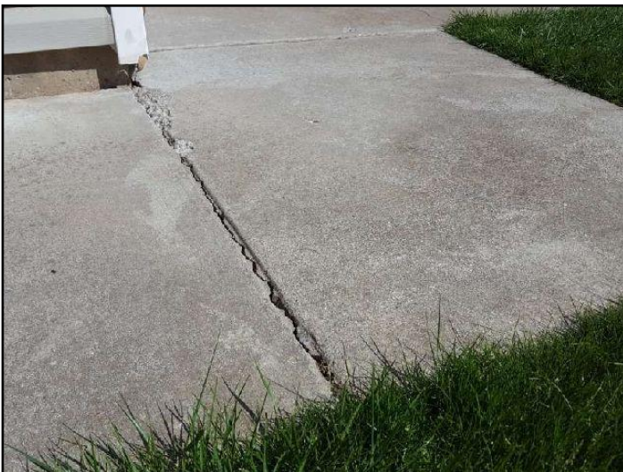
Cracked or damaged surfaces
