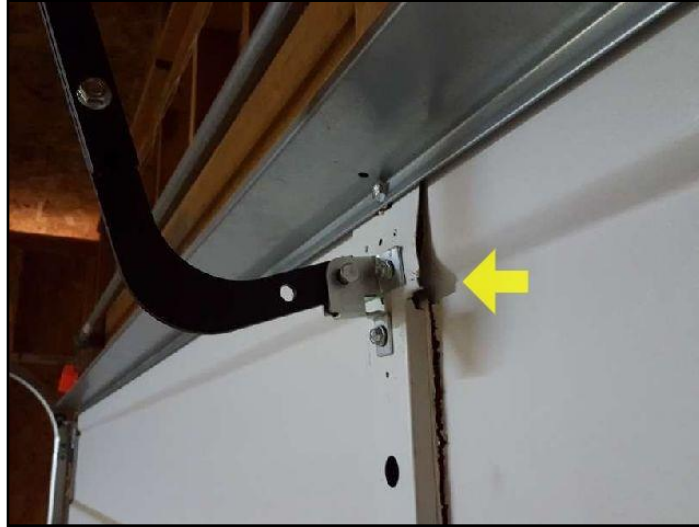
Bracket attachment damaged
