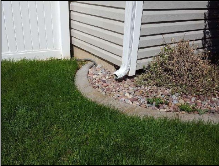
Discharge too close to building
