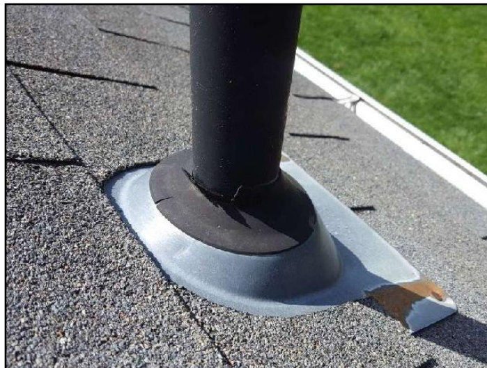
Damaged pipe/stack flashing
