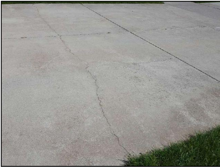
Cracked or damaged surfaces
