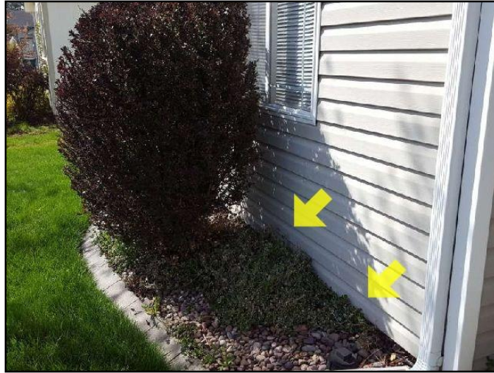
Shrubs too close to building
